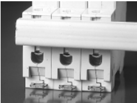
Lower terminals can be bussed together with single phase or multi-phase busbars as shown. Upper terminals can also be busbar connected.
