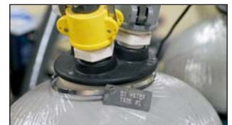
General Mechanical Identification
